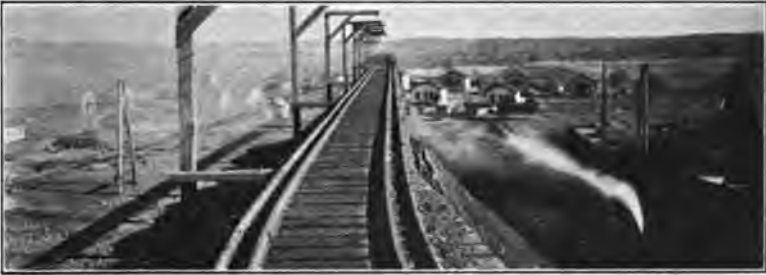
TOP OF TRESTLE SHOWING AMOUNT OF DISPLACEMENT AFTER ORE HAS BEEN LOADED.—COLBY MINE
